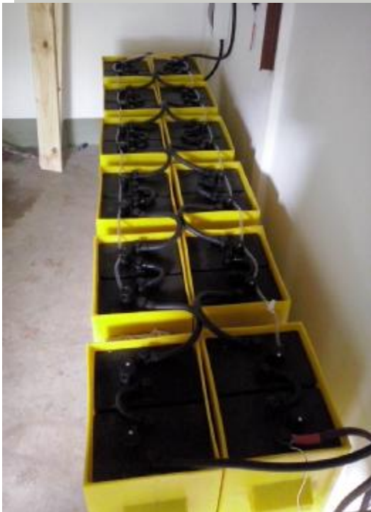
Picture 13: 1188Ah 48V FNB battery bank installed with an automatic battery filling system from Germany
